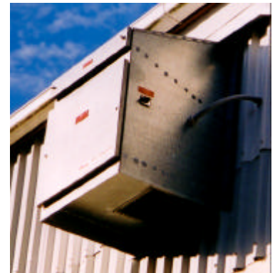
Wall mounted exhaust air handler
